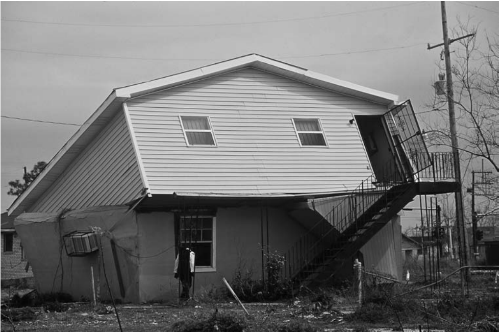
Figure 9.3 New Orleans: One of the houses overturned by a surge of water from the collapsed floodwall of the Industrial Canal during Hurricane Katrina, August 2005. This is in the Lower Ninth Ward, where flooding was deep and widespread, and almost no houses escaped damage. Photograph taken in 2007.
